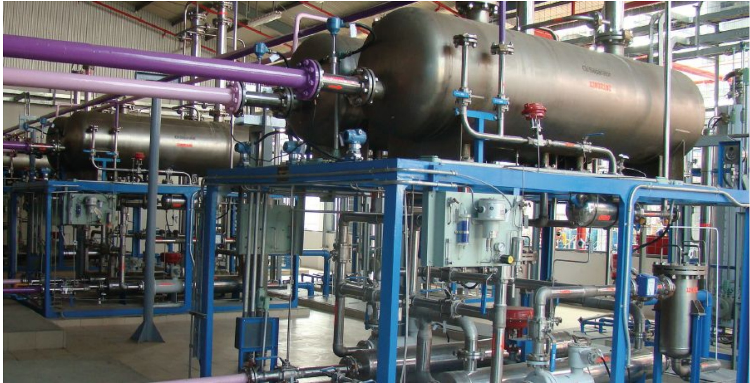
Gas separation skid with lye pumps and coolers.
